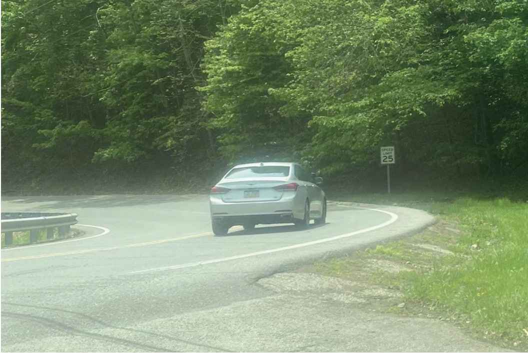
Exposed pavement edge on the outside of curve near Myrtle Hill Road
