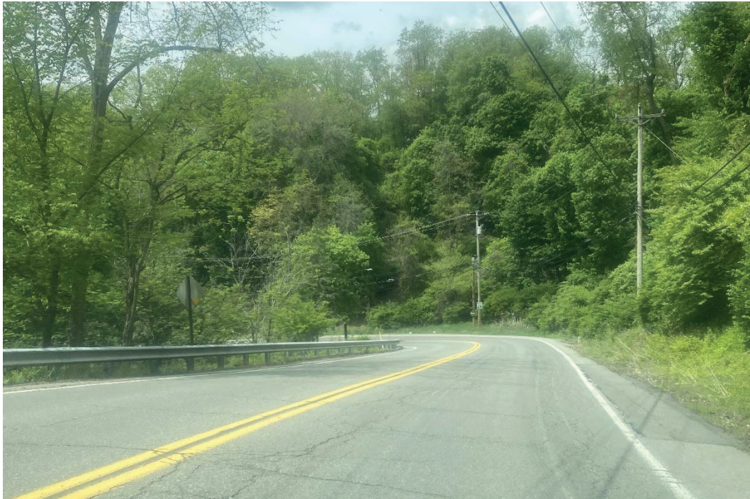
Cracked, distressed pavement on Camp Meeting Road
