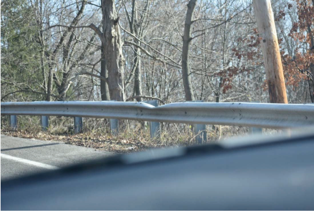
Damaged guide rail. Also, potential fixed object hazards behind the guide rail within the deflection distance.
