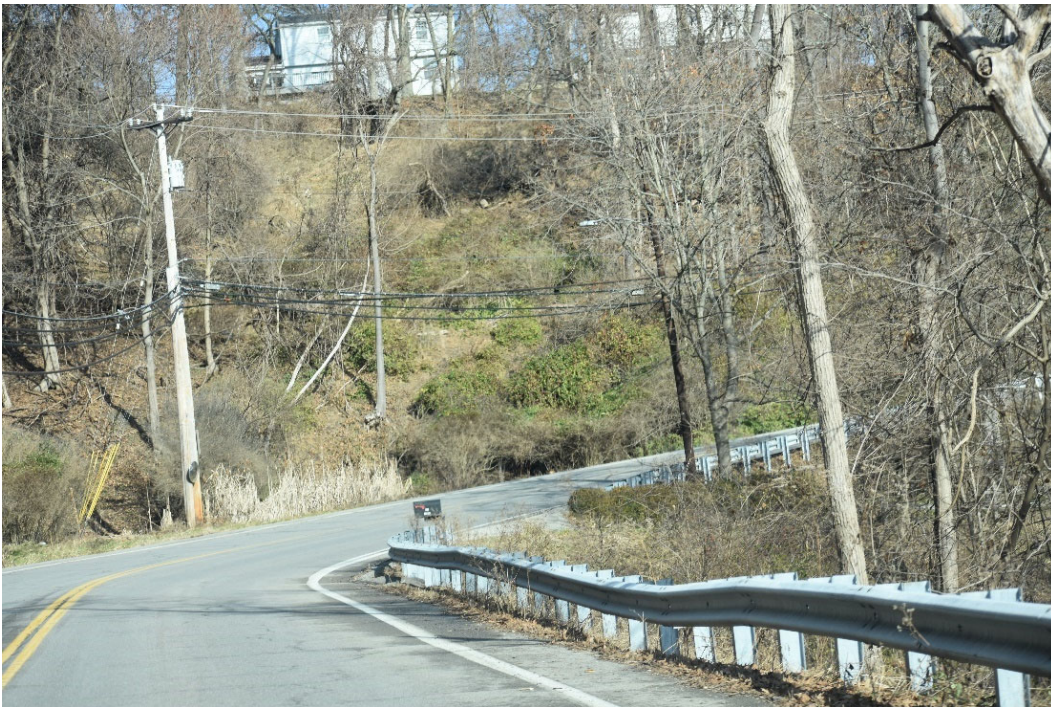
Photo shows sliding guide rail, likely due to earth sliding behind it.
