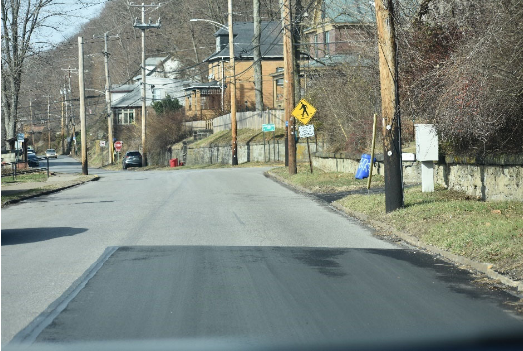
Photo shows skew in Beaver Street at its intersection with Camp Meeting Road. It also shows the lack of pavement markings.
