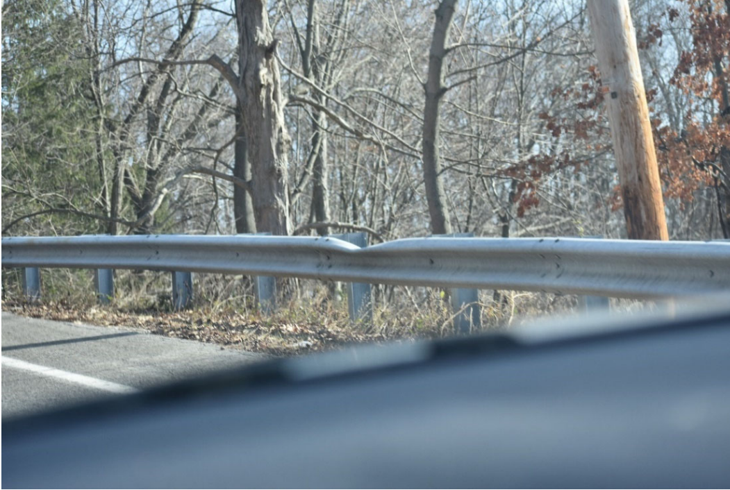
Damaged guide rail. Also, potential fixed object hazards behind the guide rail within the deflection distance.
